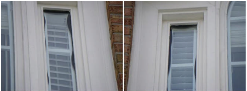
Master bedroom fixed side windows are defective. See photo. Monitor conditions. Replace as needed.
