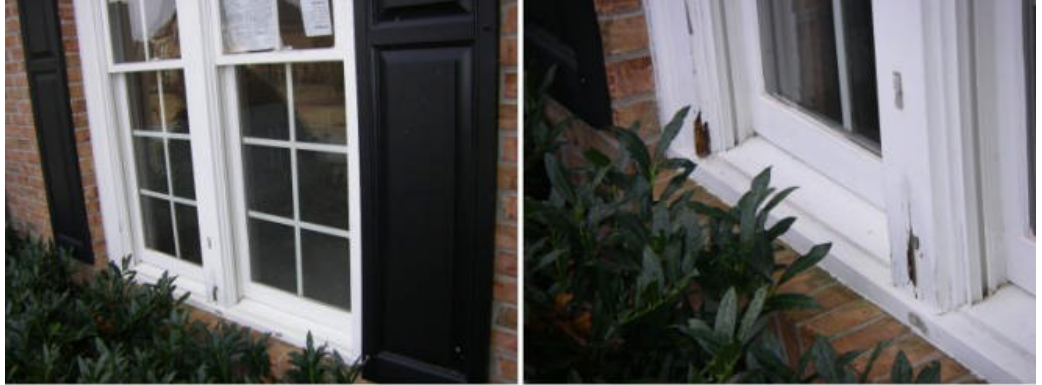
Water damage was noted in the dining room window trim. See photos. Repairs are needed.
