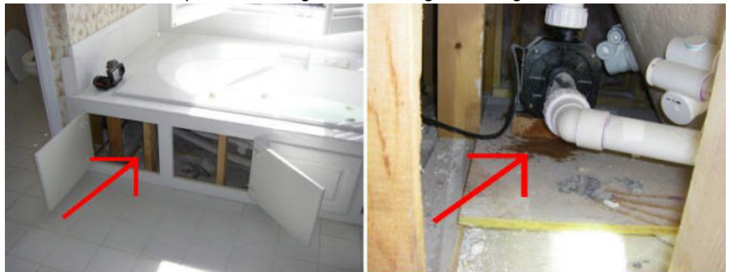
The jetted tub is leaking near the motor. See photo. Repairs needed by a qualified plumber.
