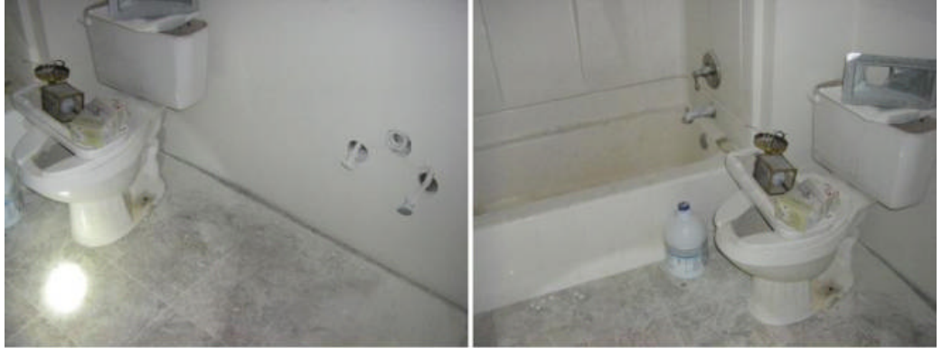
The basement bath has not been completed. Not tested.
