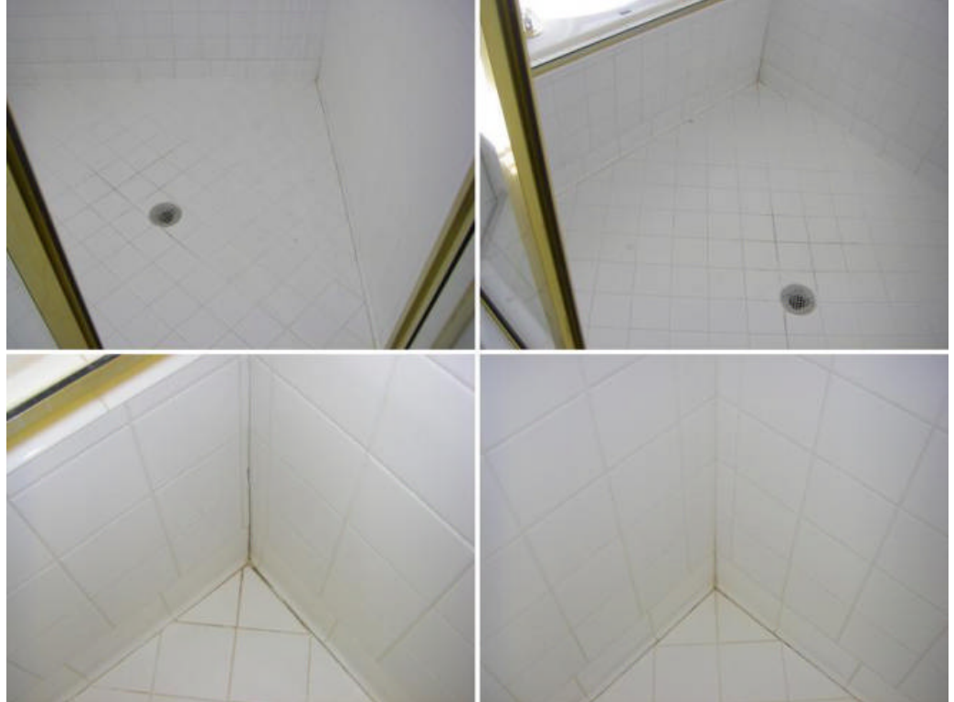
Budget for improving the caulking and grouting in the master bath shower stall around the drain and sides to prevent leaking into the ceiling or framing below.
