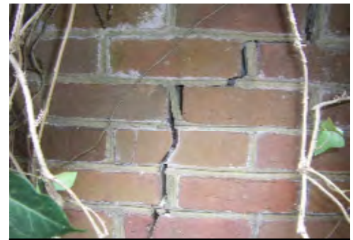
Displacement in the left retaining wall
