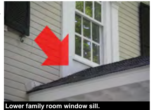
Lower family room window sill.
