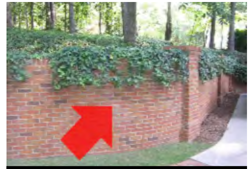
Right retaining wall. Displacement
