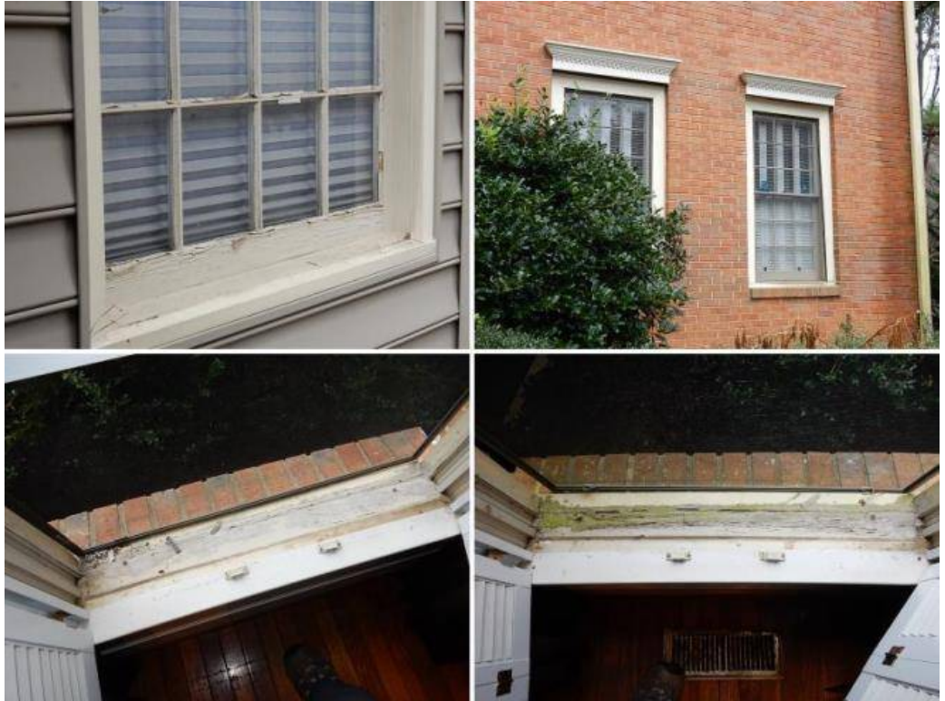
The sash springs are not connected in several window units. Repair needed.
