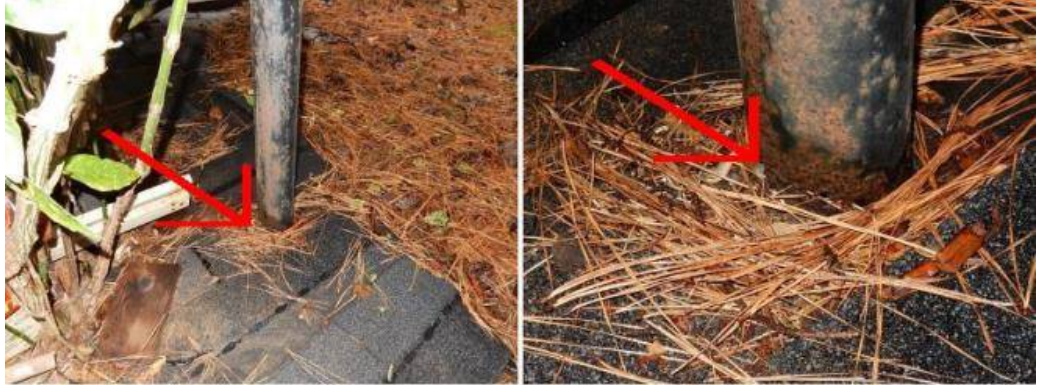
The base of the steel columns are rotting. Unsafe condition noted. Budget for replacement ASAP. See photo.
