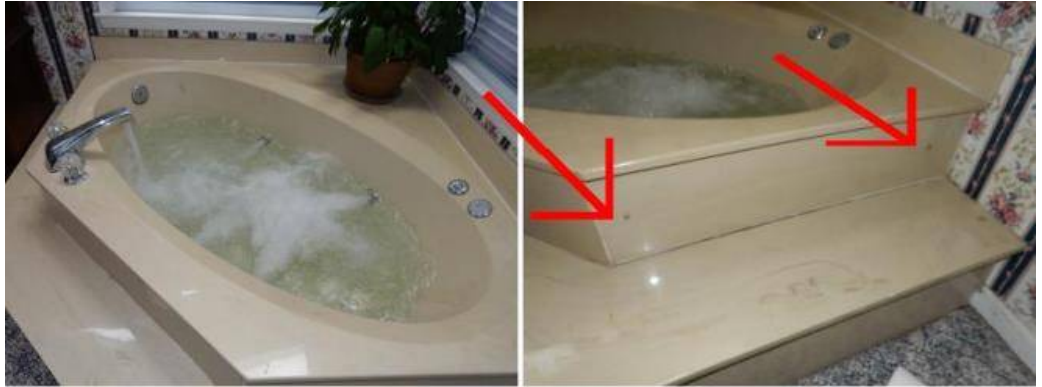
Master bath jetted tub appears to be functioning as intended. Budget for servicing. Could not remove the access panel to the jetted tub motor for inspection. See photo. Removing may damaged the caulking.
