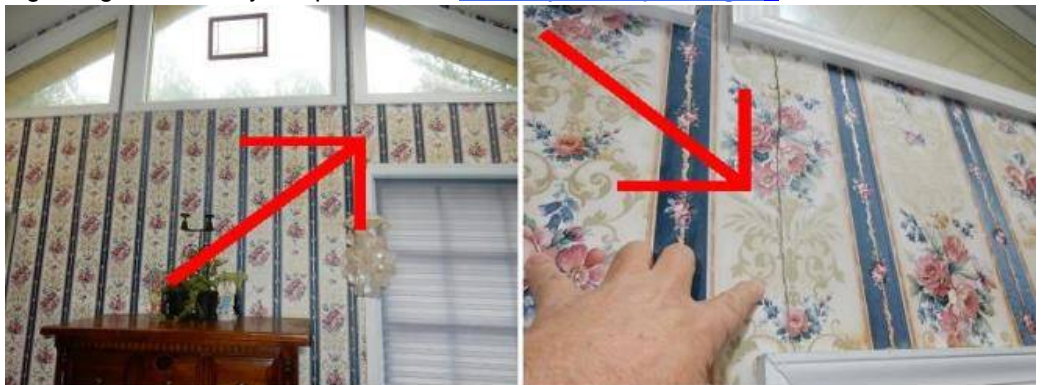
Displacement crack noted in the drywall in the master bath. See photo. Could not determine the cause. Further investigation needed.
