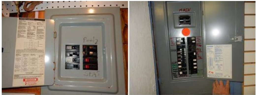
Main disconnect panel is located in the basement.
