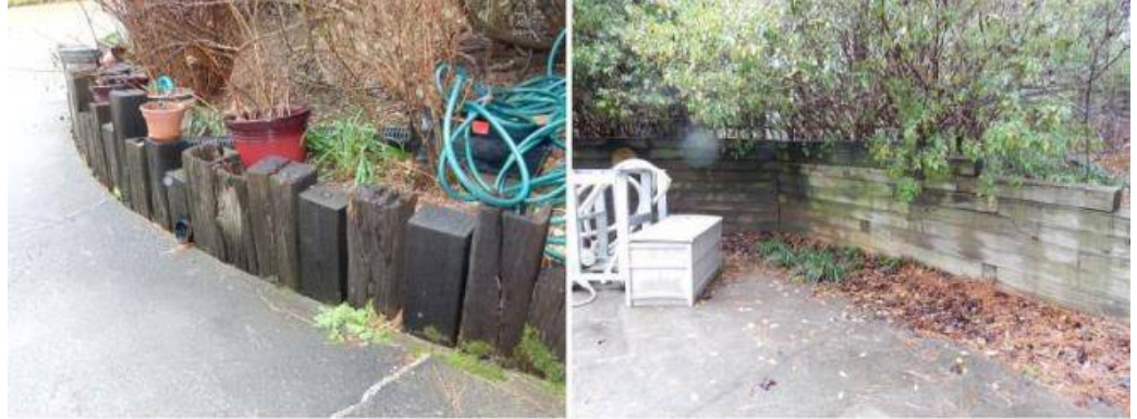
Crosstie retaining wall noted at the driveway. Wood (landscape timber) retaining wall noted pool.
