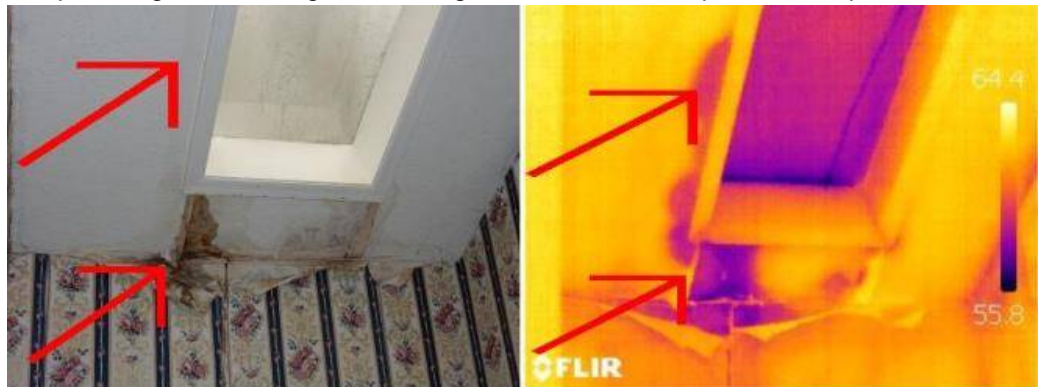
Active leaking noted at the master bath skylight flashing. See Infrared photo. A licensed roofing contractor should be called to make further evaluation and repairs as needed.
