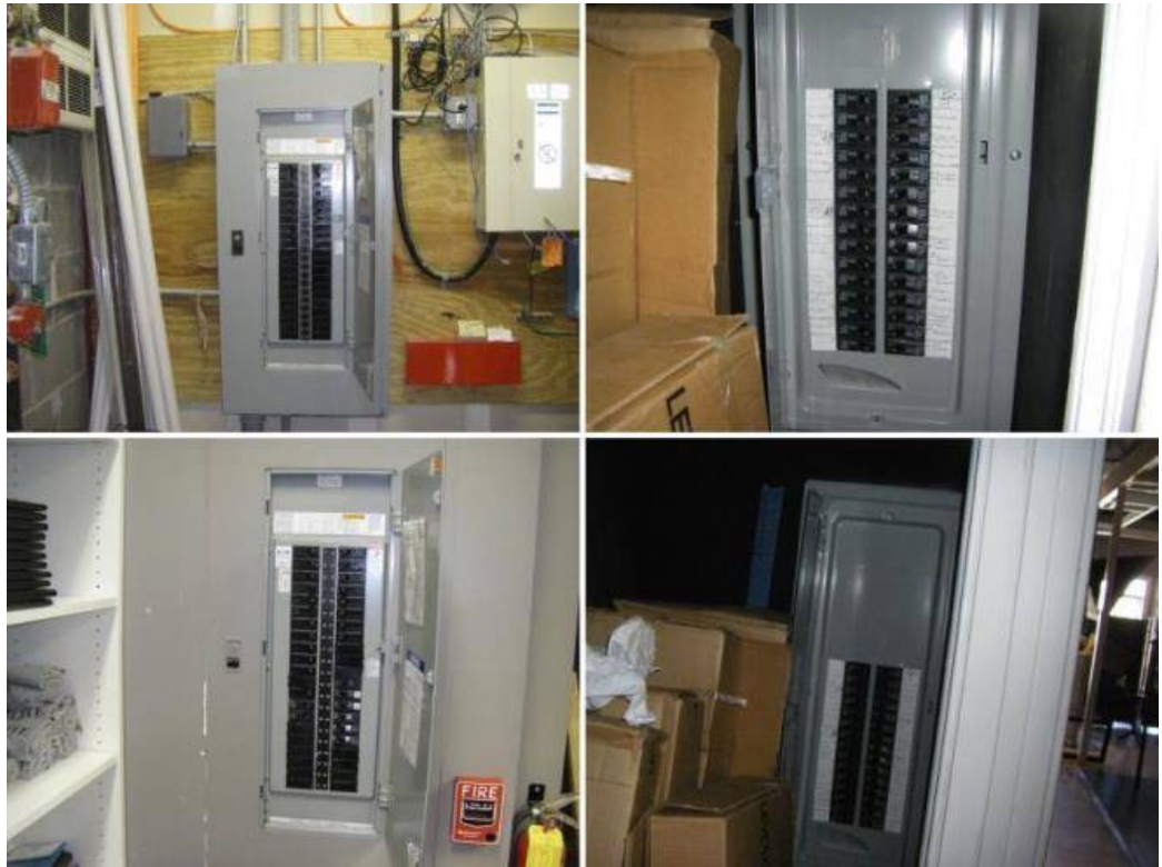
Main disconnect panels are located in the utility areas.
