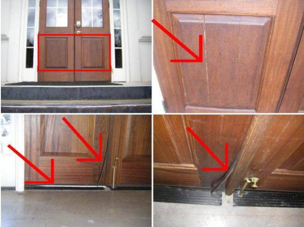
The main entrance door on the south side of the building is in poor condition. Budget for repairs or possible replacement. The panels are cracked. The weatherstripping is in poor condition. Air gap noted under the door. See photo.
