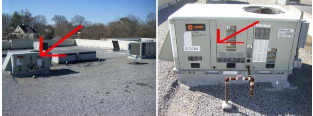
The unit for the top floor south east corner of the building is not functioning as intended at this time. This unit should be serviced by a qualified HVAC contractor. See photo.
