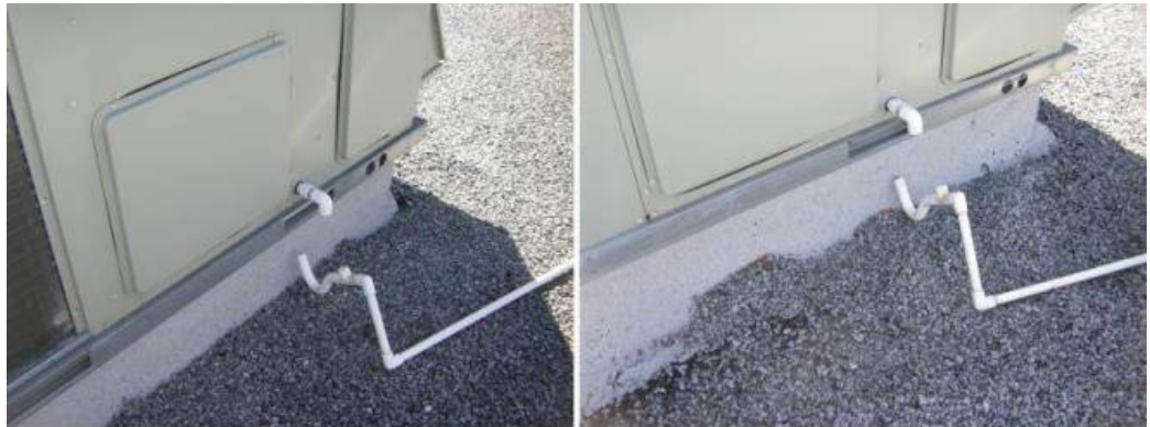
The condensation drains are not connected to the roof top units. Correction is needed by a HVAC contractor. See photo.
