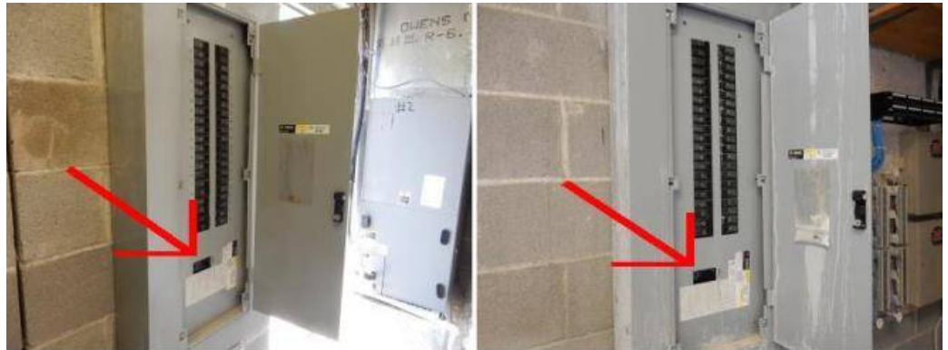
The main disconnect is located at the master panel. The size of the main electrical disconnect panels are 200 amps each. Appears serviceable where exposed for inspection. Wiring appear to be serviceable at this time where exposed for inspection.
