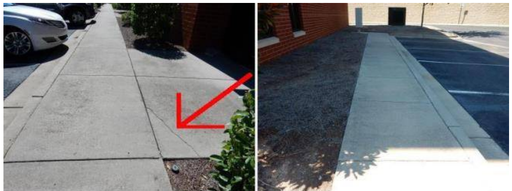
The sidewalk appears to be in good condition at this time. Cracks noted appear to be normal.
