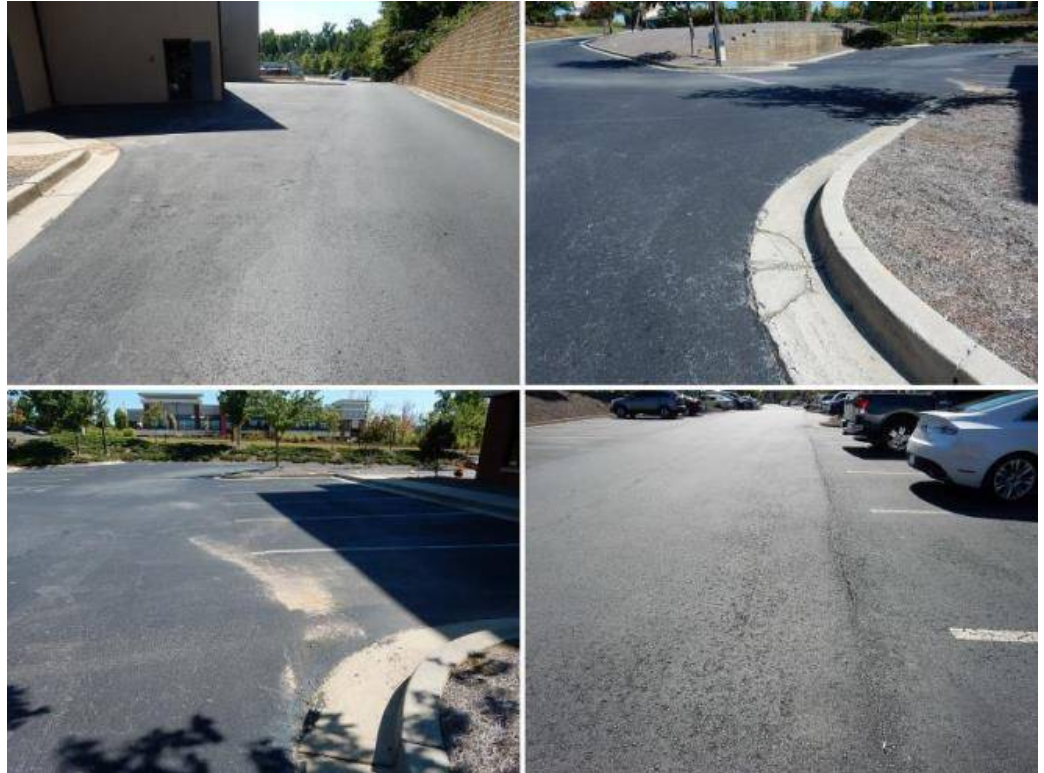
The driveway appears to be in good condition at this time. Cracks noted appear to be normal.
