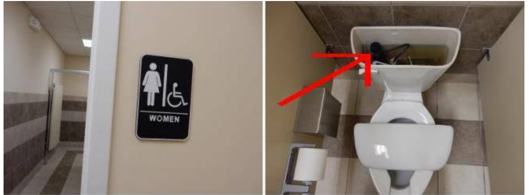
Flush valve will not turnoff in the woman's restroom, main floor.
