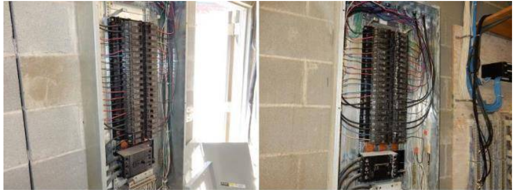
The panel was accessible and the panel cover was removed. The electrical disconnects are breakers.
