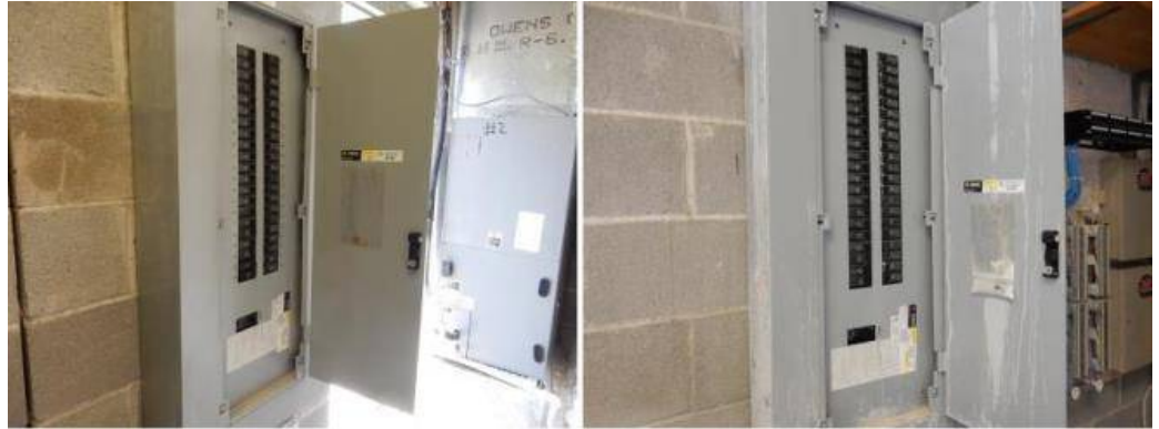
Main disconnect panels are located in the utility rooms.
