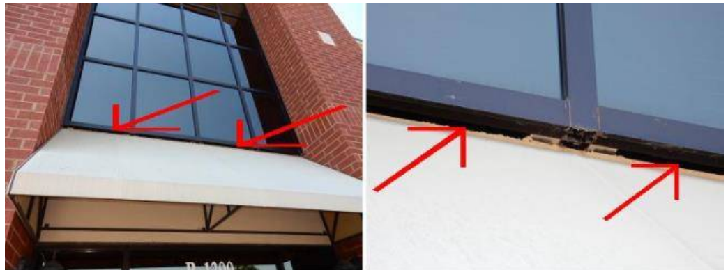
The gap above the front entrance awning should be filled to prevent insects from entering the wall or building. See photos.
